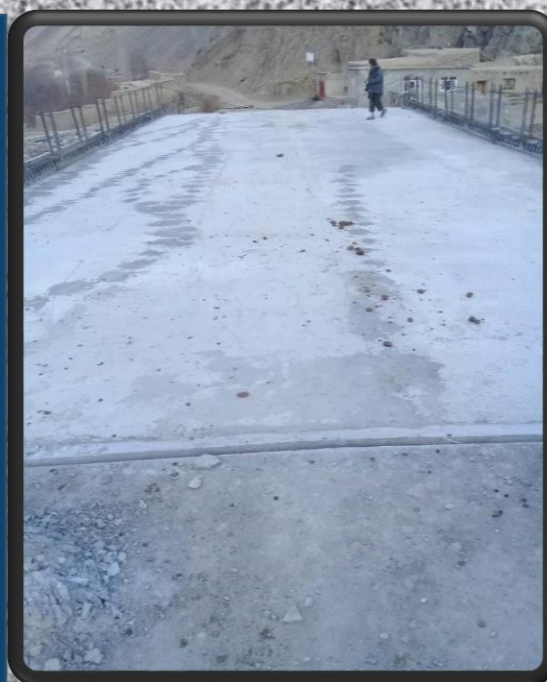
Construction of 40 Rm Bridge in Guzargah Noor District of Baghlan Province by NRAP MoPW
