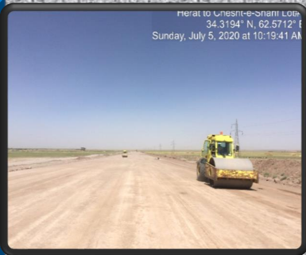
Construction of 35 km road in Chesht Sharif of Herat Province through NRAP
