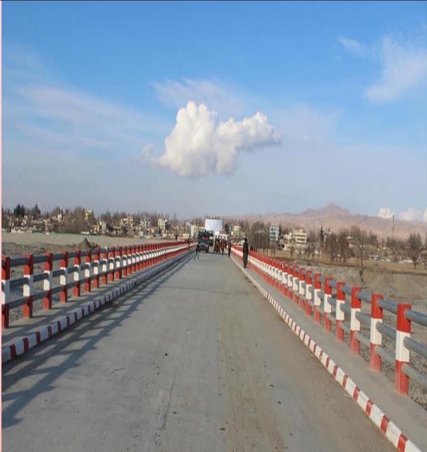
Construcion of 200 Rm Bridge in Taliqan district of Takhar Province by NRAP.MRRD
