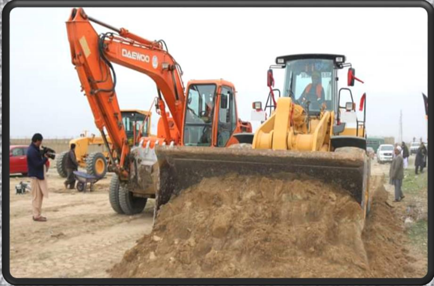
Construction work of 5.76 km road from Bazar sar dawra to Central Airport of Kunduz Province by NRAP.MRRD
