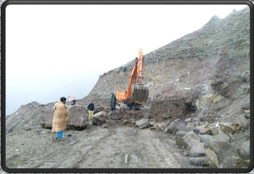
Construction work of 25.8 km road in Kamdesh District of Nooristan Province by NRAP.MRRD
