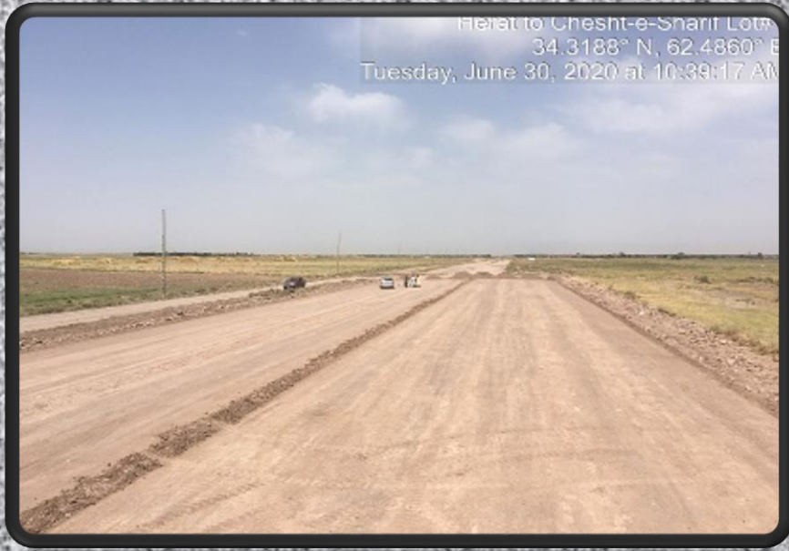
Construction of 35 Km road (lot#1) in chesht District of Herat province by NRAP. MoPW
