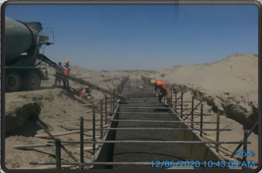
Construction work of 300 Rm Bridge along Zaranj to Kang road Kang district of Nimroz Province by NRAP. MoPW
