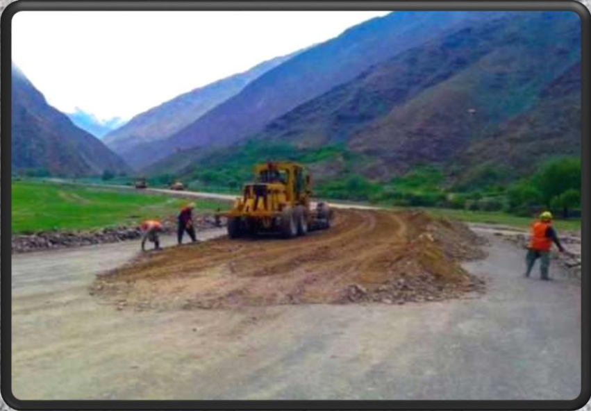
Construction work of 15 km road from Farkhar District to Warsaj of Takhar Province by NRAP. MoPW
