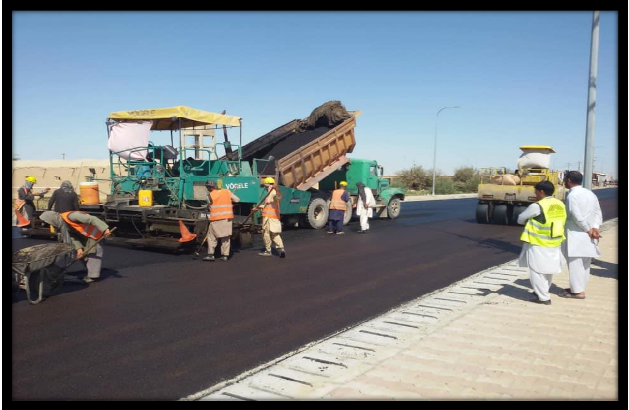
Construction of 7.2 km road in Qurghan district of Faryab Province by NRAP.MoPW
