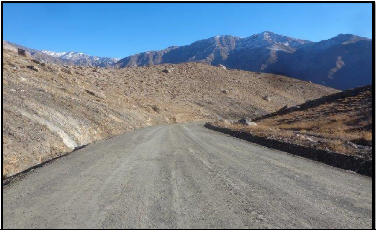
Construction of 10.6 Km of gravel surface road from center of Rukha district to Doshakh, Panjshir province
