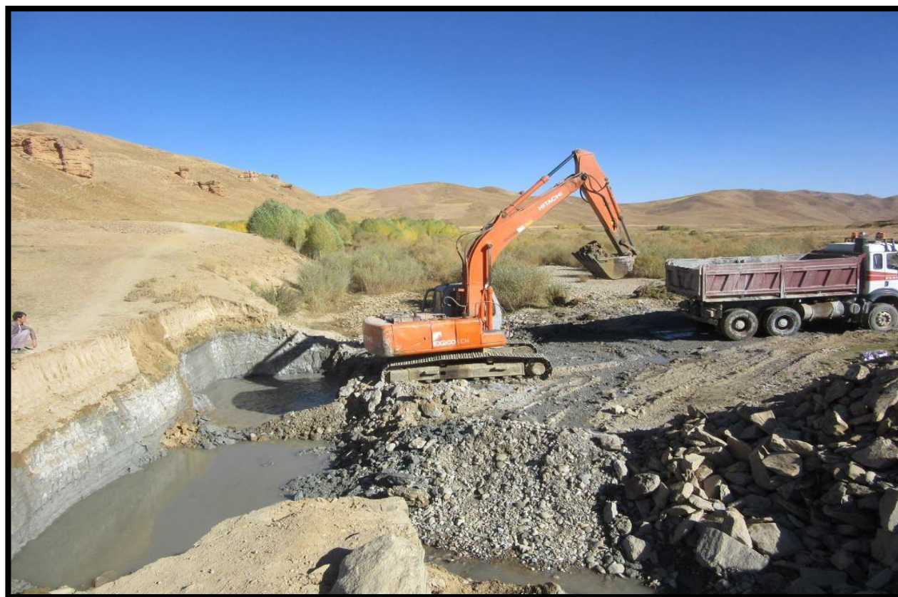
Initiation of 15 running meters bridge along with its joint road in Dane Qhamoghe village, lalwa-Sarjangal district of Ghor Province.
